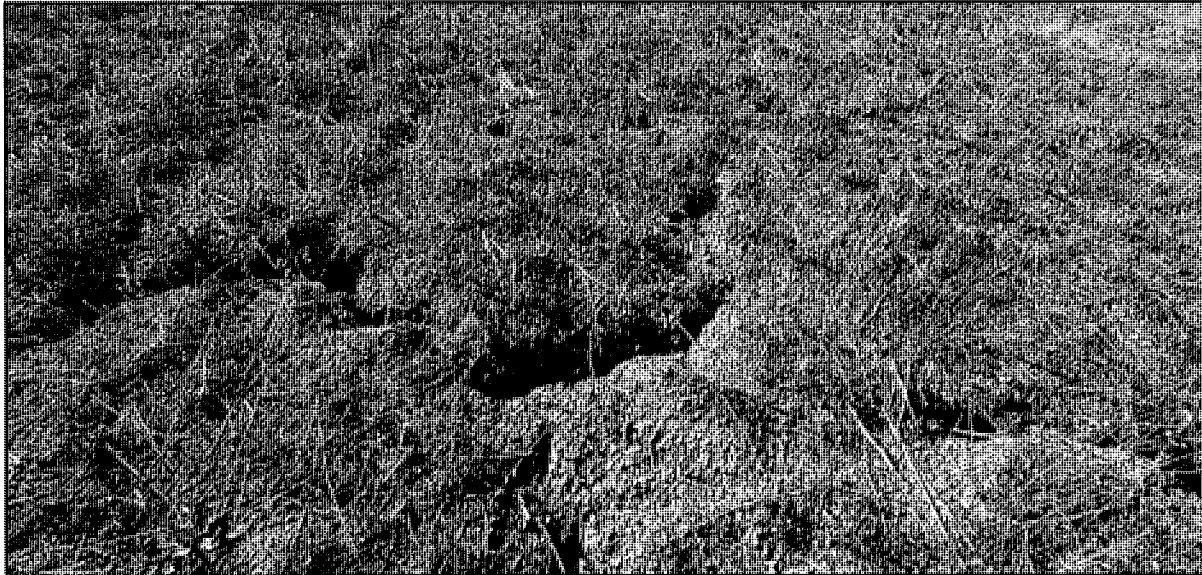
Small Fissures and Cracks Example of Cracking Throughout the Site
