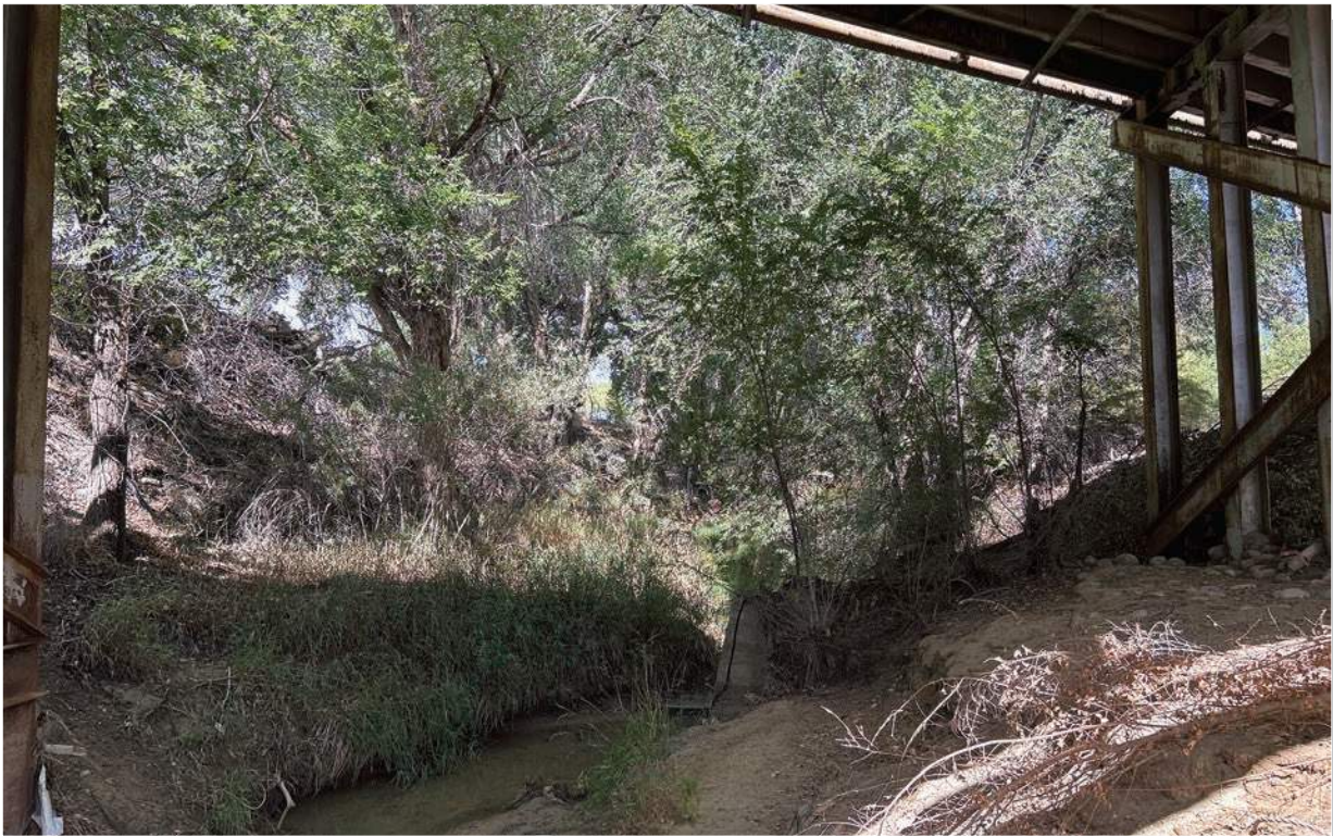
Photo 4 - Eroded banks and grading under CR 3500. View is north.
