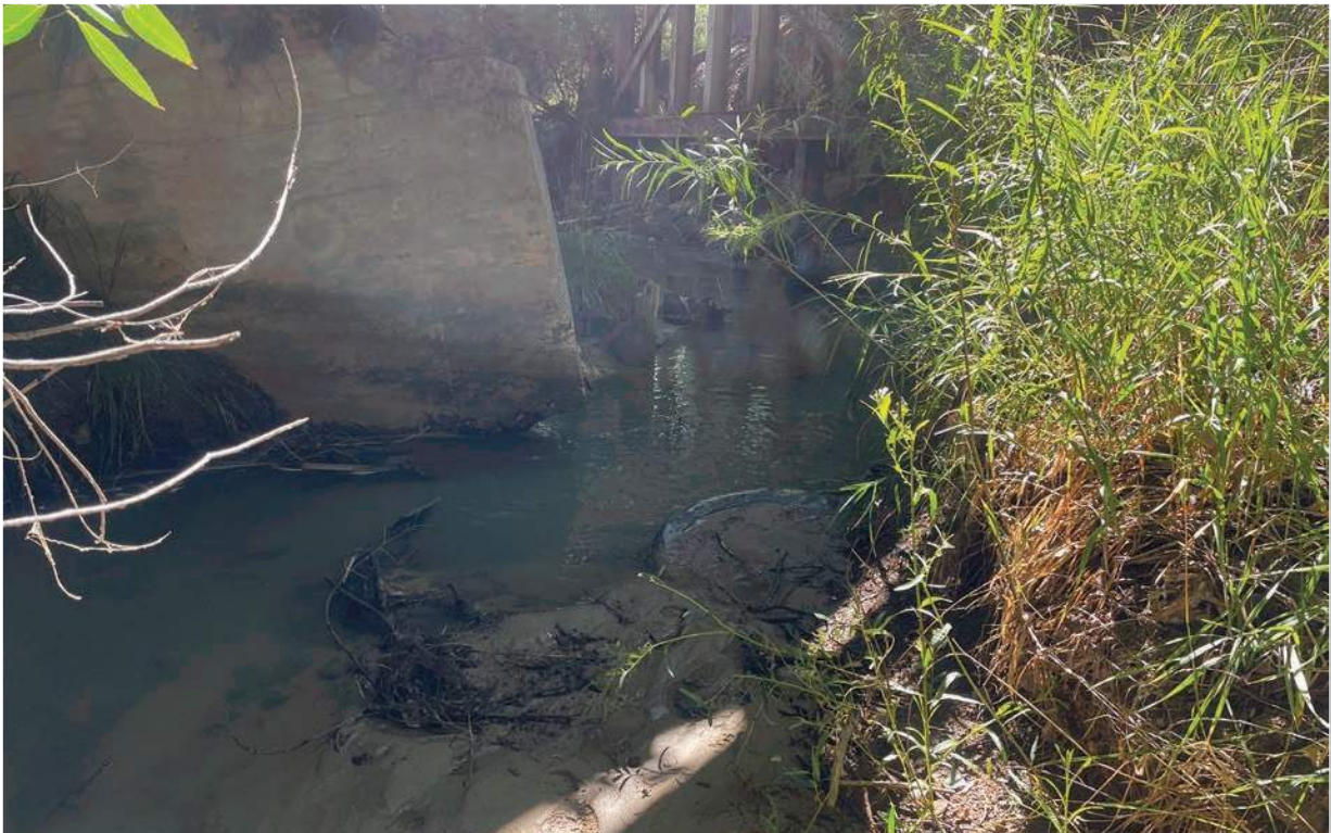
Photo 2 - Concrete pylons under CR 3500 with heavy erosion and channel alteration. View is north.
